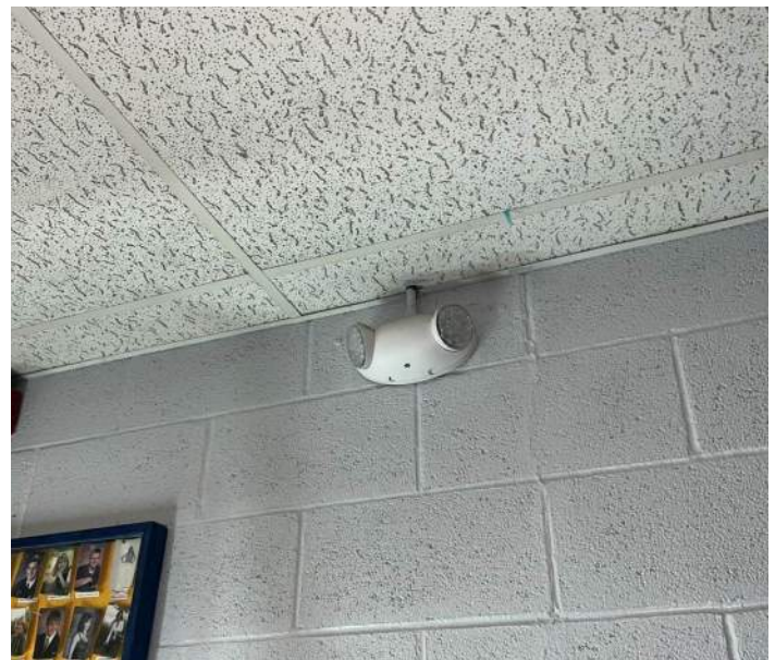
EMERGENCY LIGHTING UNIT
