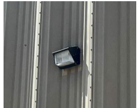
TYPICAL EXTERIOR WALLPACK ON THE 1978 BUILDING
