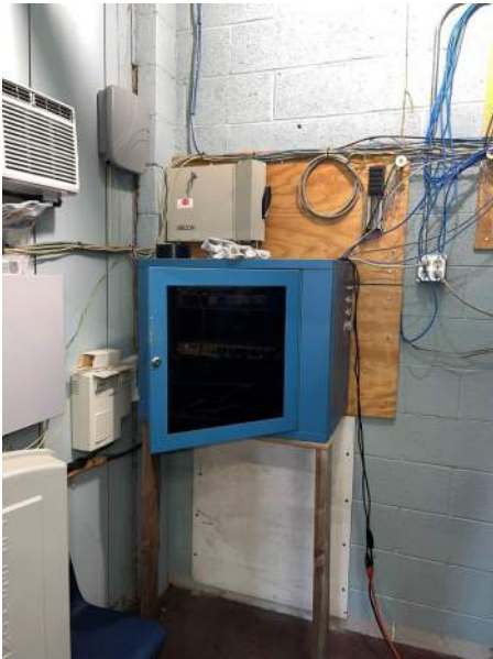
HIGH SCHOOL DATA ROOM WITH WALL RACK
