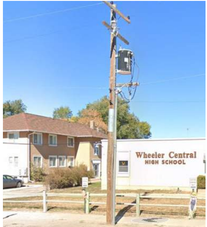
HIGH SCHOOL POLE MOUNTED TRANSFORMER
