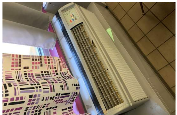
SHOP CLASSROOM PTAC
