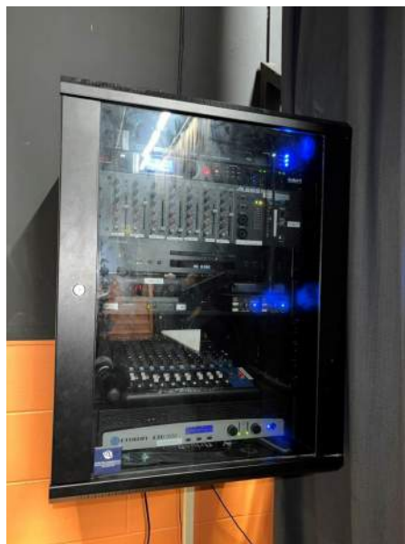
EXISTING AUDIO EQUIPMENT RACK IN THE 1978 BUILDING
