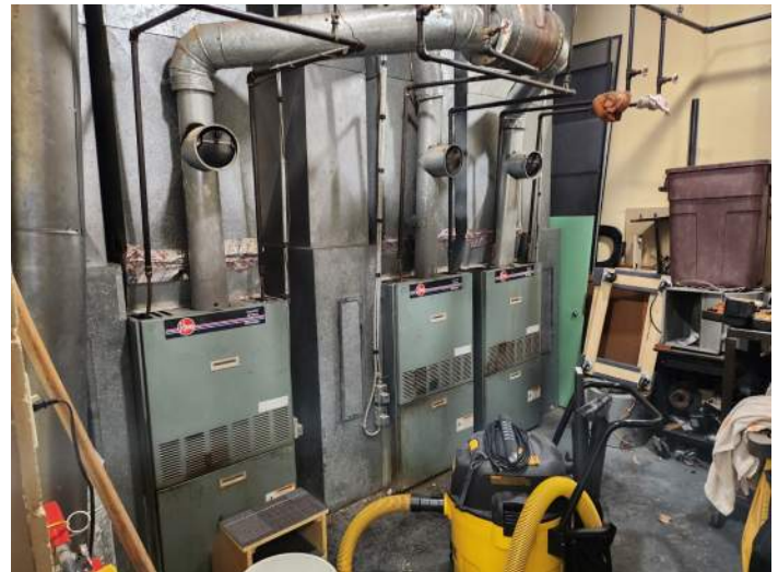
1978 CLASSROOM AND CAFETERIA DIESEL FURNACES
