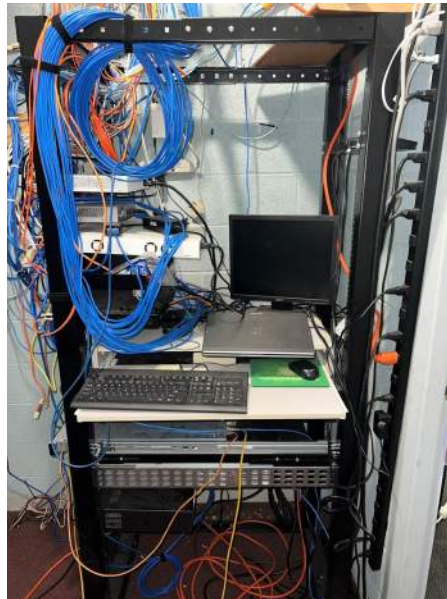
FLOOR MOUNTED RACK
