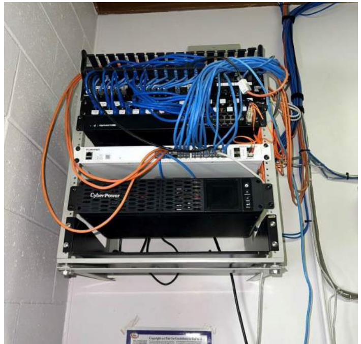
EXISTING DATA RACK IN THE 1978 BUILDING
