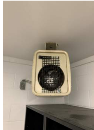
ORIGINAL LOCKER ROOM HEATER
