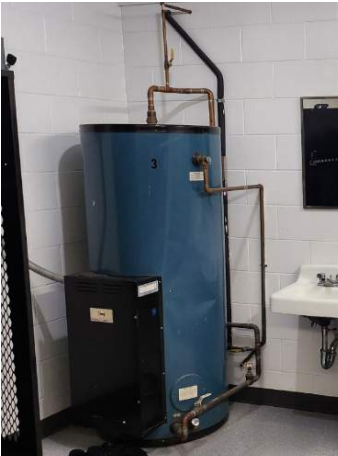
ORIGINAL 1978 GYM WATER HEATER
