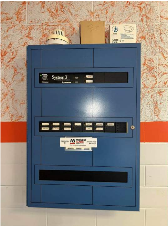
HIGH SCHOOL FIRE ALARM PANEL
