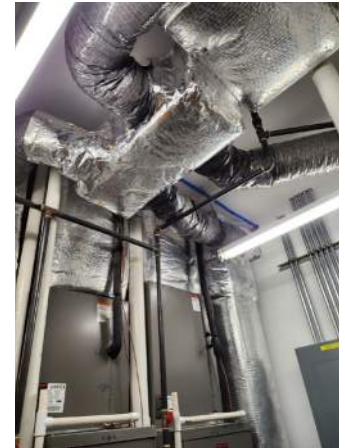
FRESH AIR DUCTWORK SERVING 2010 BUILDING
