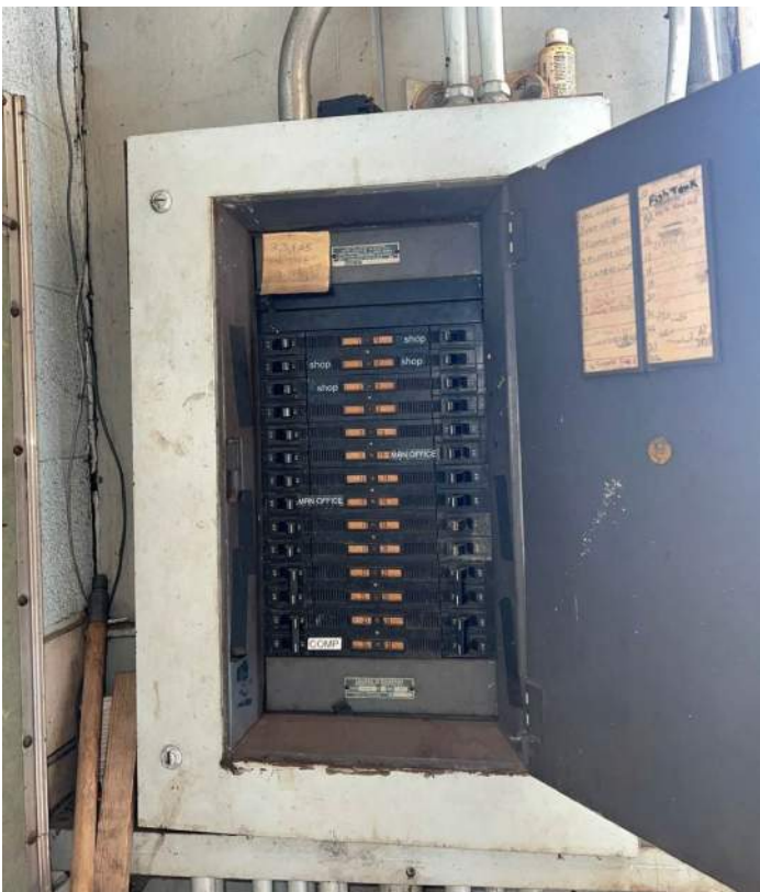
HIGH SCHOOL TYPICAL PANELBOARD
