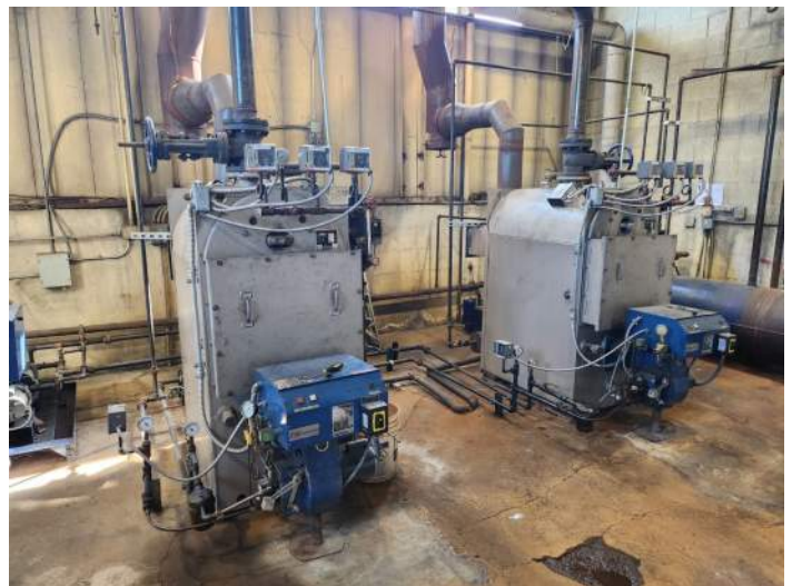
LOW-PRESSURE STEAM BOILERS
