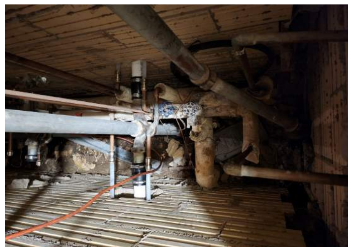
SHOP CLASSROOM PTAC
