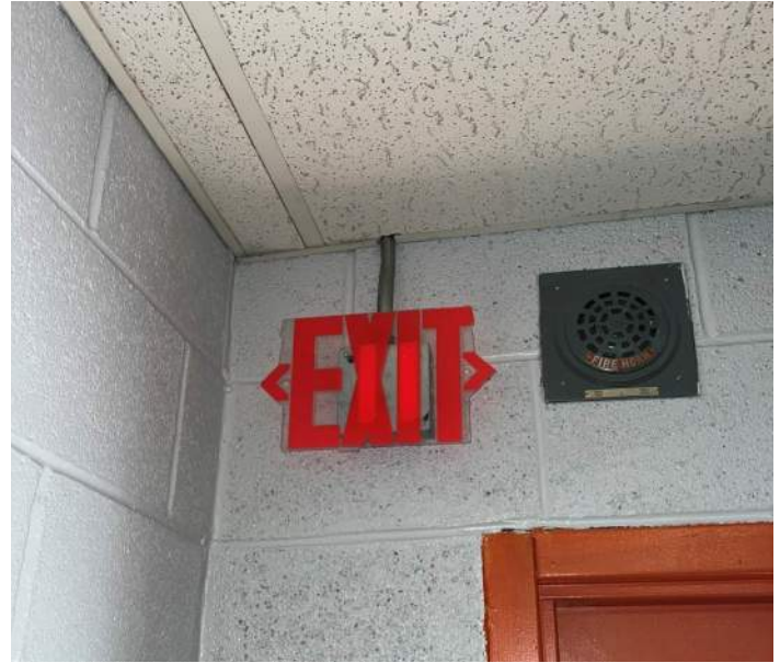
NON-ILLUMINATED EXIT SIGN
