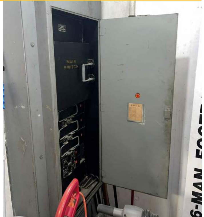
OLD GYM DISTRIBUTION PANEL
