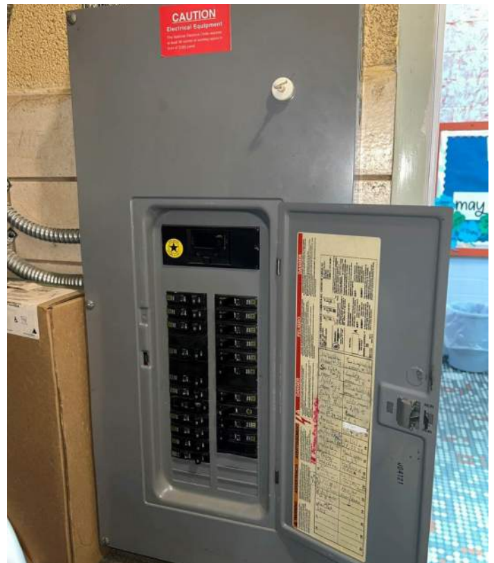
ADDED LOAD CENTERS
