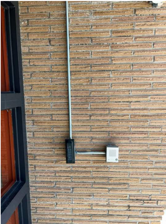
HIGH SCHOOL ENTRY ACCESS CONTROLS
