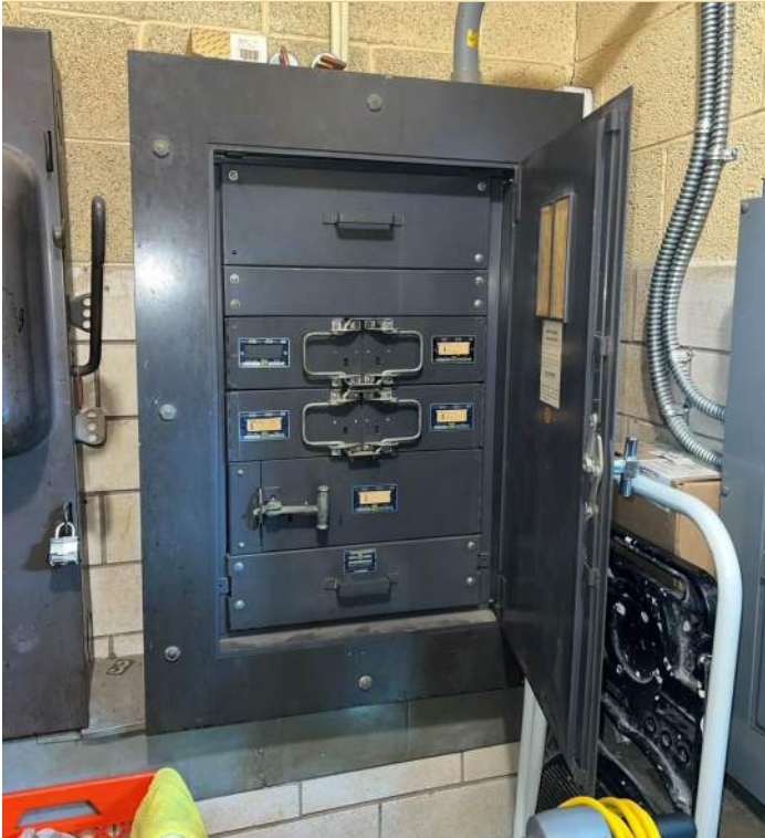
HIGH SCHOOL DISTRIBUTION PANEL
