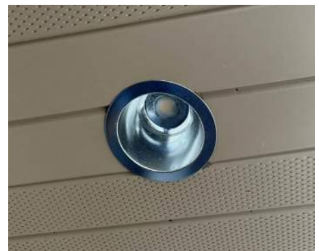
RECESSED DOWNLIGHT ON THE 2010 BUILDING
