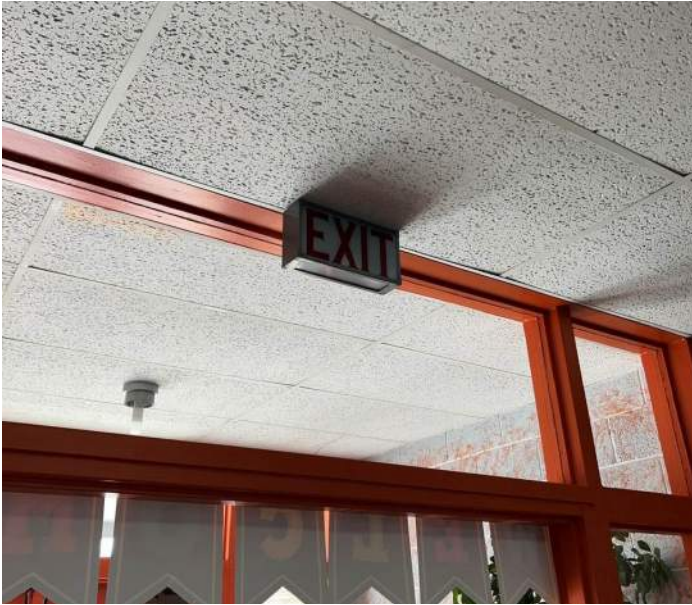
HIGH SCHOOL ILLUMINATED EXIT SIGN
