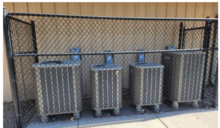
CONDENSING UNITS SERVING 2010 BUILDING
