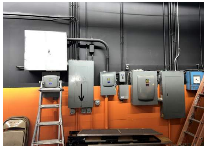
NEW GYM BUILDING MAIN DISCONNECTS
