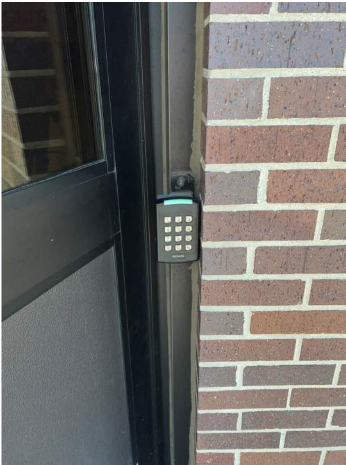
NEWER CARD READER AT AN EXTERIOR DOOR AT THE 1978 BUILDING
