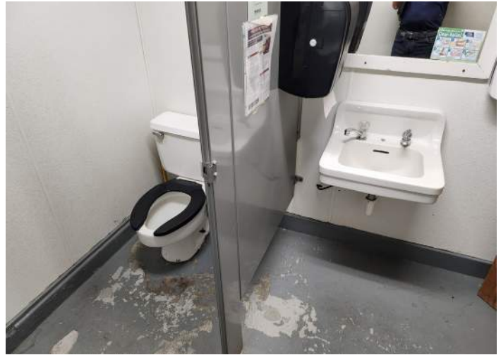
GYM RESTROOM FIXTURES
