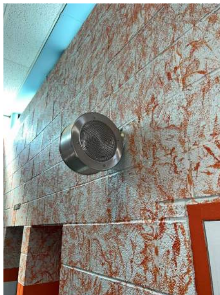
HIGH SCHOOL TYPICAL CORRIDOR PAGING SPEAKER
