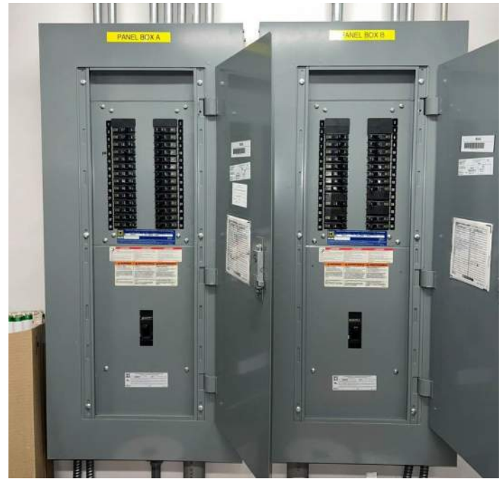
2010 ELEMENTARY SCHOOL BUILDING ELECTRICAL SERVICE ENTRANCE EQUIPMENT
